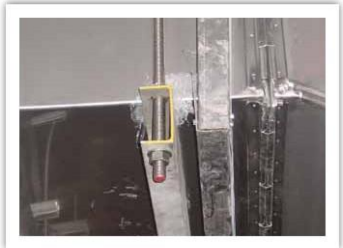
Appropriate hanger support require for the ductwork system
